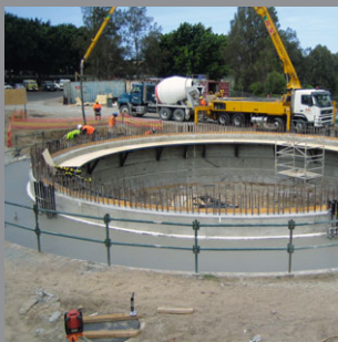
Sewage water reservoir Brisbane (AU), 2007
