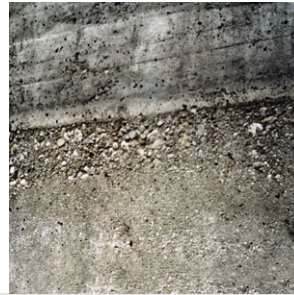
Results of abrasion and acid attack in a sewage treatment plant
